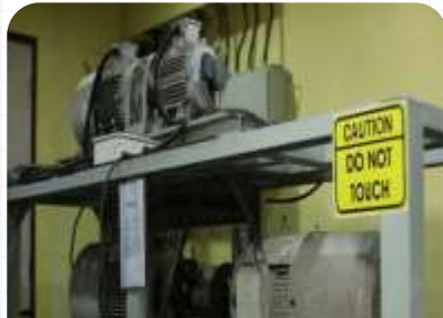
POWER ELECTRONICS LAB
